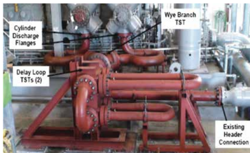
Figure 18: Early example of a combination PAN Manifold and PAN filter retrofitted to an existing 1000-rpm compressor in 2009.
